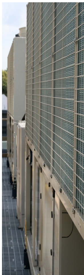
Side view on the platform of the two McQuay 500 Kva chillers at the new R1 data centre
