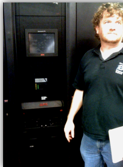
Andrew Munsie-Data Centre Manager beside IT UPS Management console in the new R1 Data Centre
