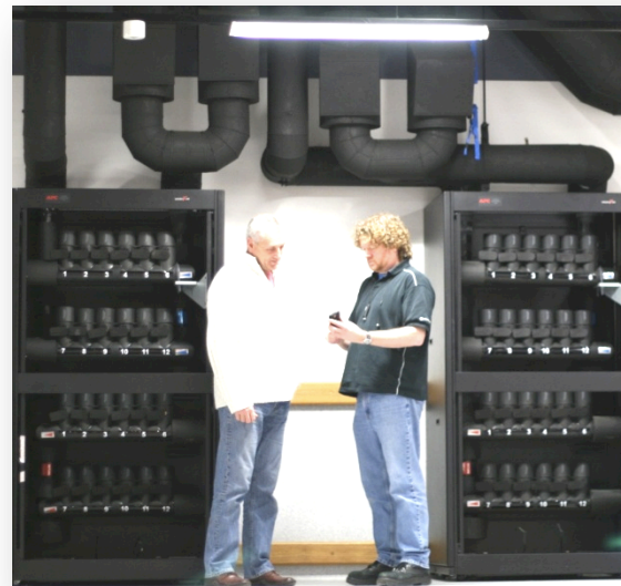
Project manager, Nick Stace, and Data Centre manager, Andrew Munsie, alongside two of the four CDU water distribution units in the West Hall of the new R1 data centre
