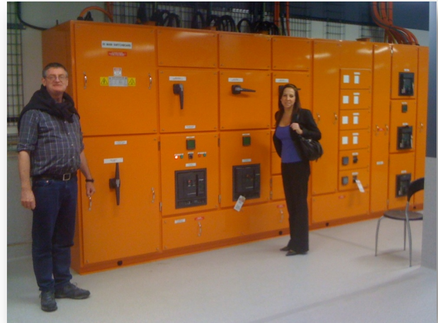
Richard Smith-Production Services Manager and Jennifer Hogan-Dell Customer manager, in front of main switchboard in new R1 Data Centre
