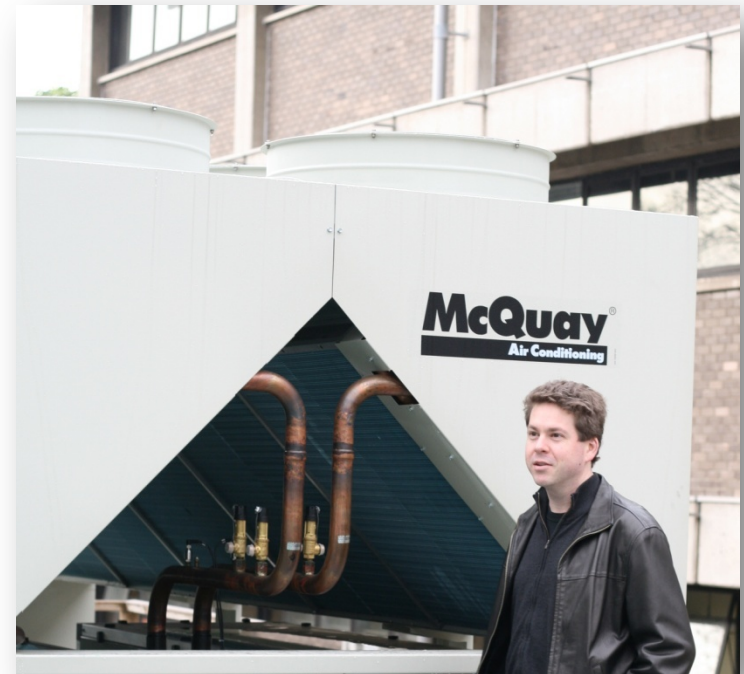
Toby Harrison-Infrastructure Project Manager alongside one of the two 500Kva McQuay air cooled chillers outside the rear of new R1 data centre
