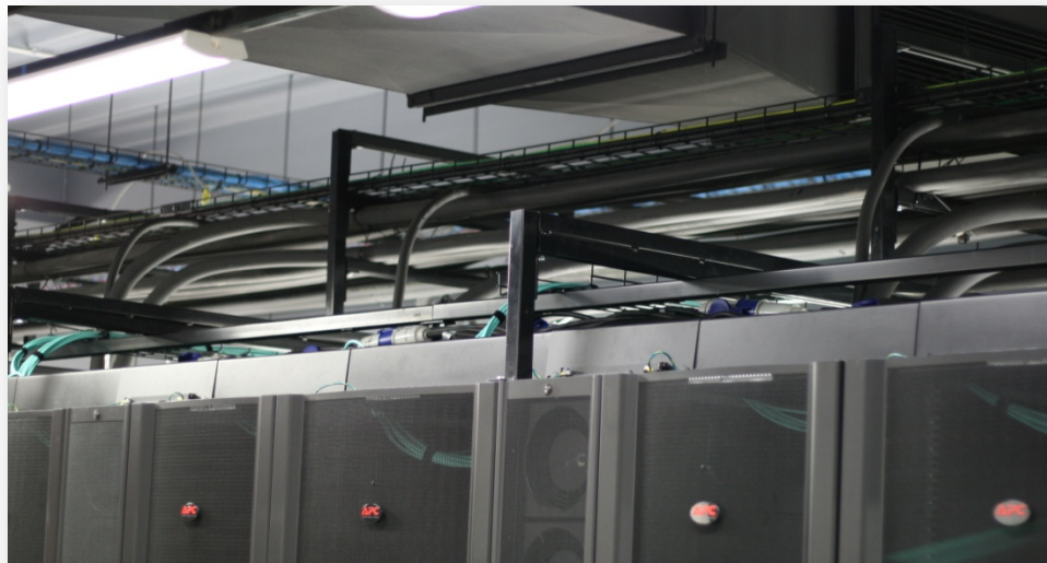
Overhead structured cabling of fibre and minimal UTP as used in the new R1 data centre
