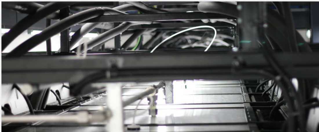
Overhead cabling and water distribution above POD A in the West Hall of the new R1 data centre
