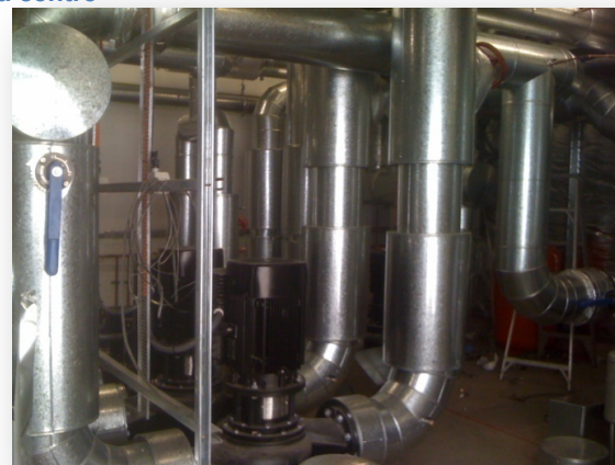
Pumps and distribution pipes in the plant room of the new R1 data centre
