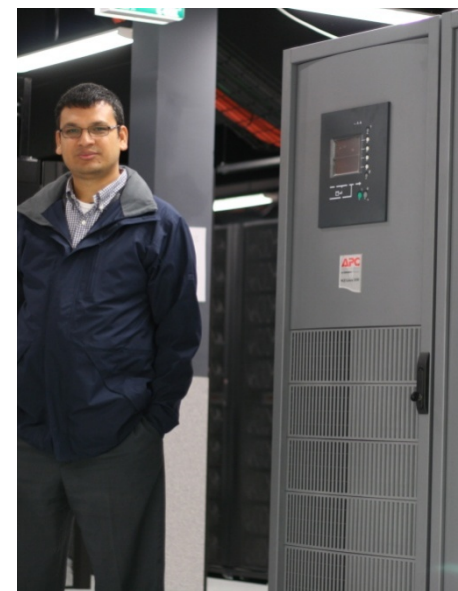
Sudeep Joshi-Infrastructure Design & Capacity Manager beside the Mechanical UPS battery bank in the new R1 Data Centre
